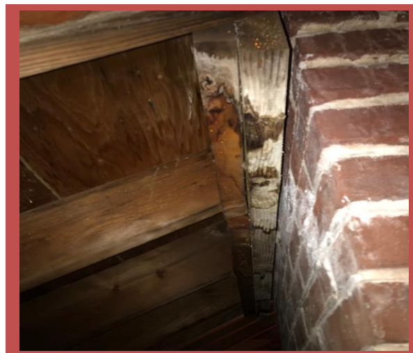
Attic water damage.
